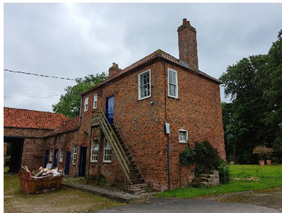
View of main building indicating cumbersome external timber stair
